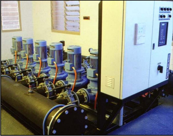
Variable Speed Booster set for town water supply
