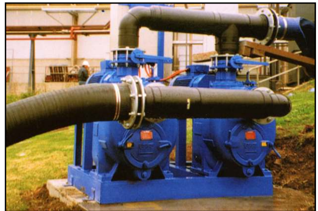
Effluent Pumping System at major Milk Factory
