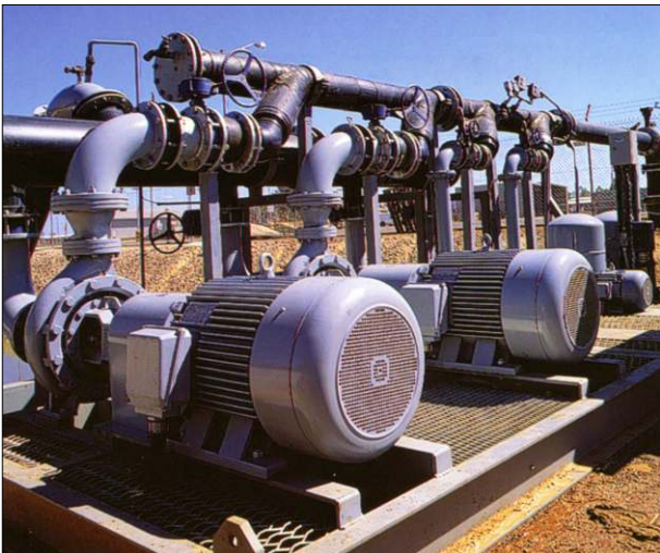
Fully Automated 5 Pump Water Supply Pumping System
