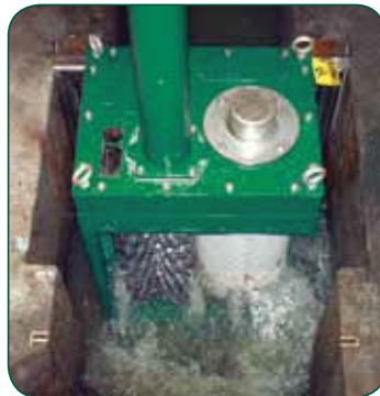
This model CMD replaced an old comminutor without reconstructing the channel.
